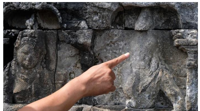
Figure 1. The damage of Candi Borobudur Source: detiktravel.com
